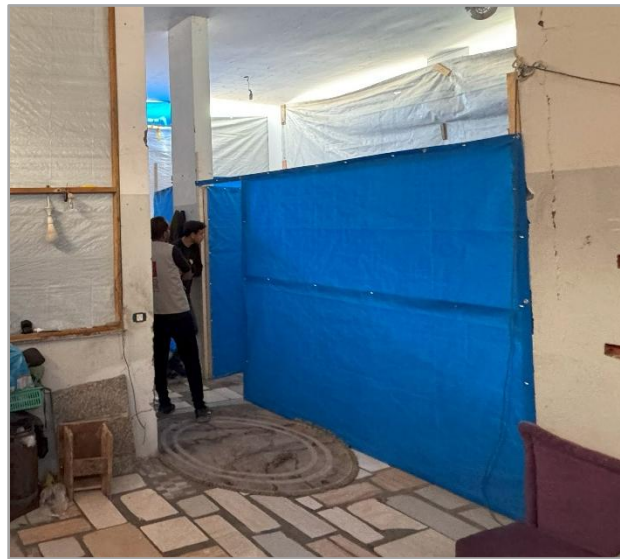
Figure 3 Internal partitioning of an open shelter using tarpaulins, with wide walkways left in between – HEKS/EPER, July 2025.
