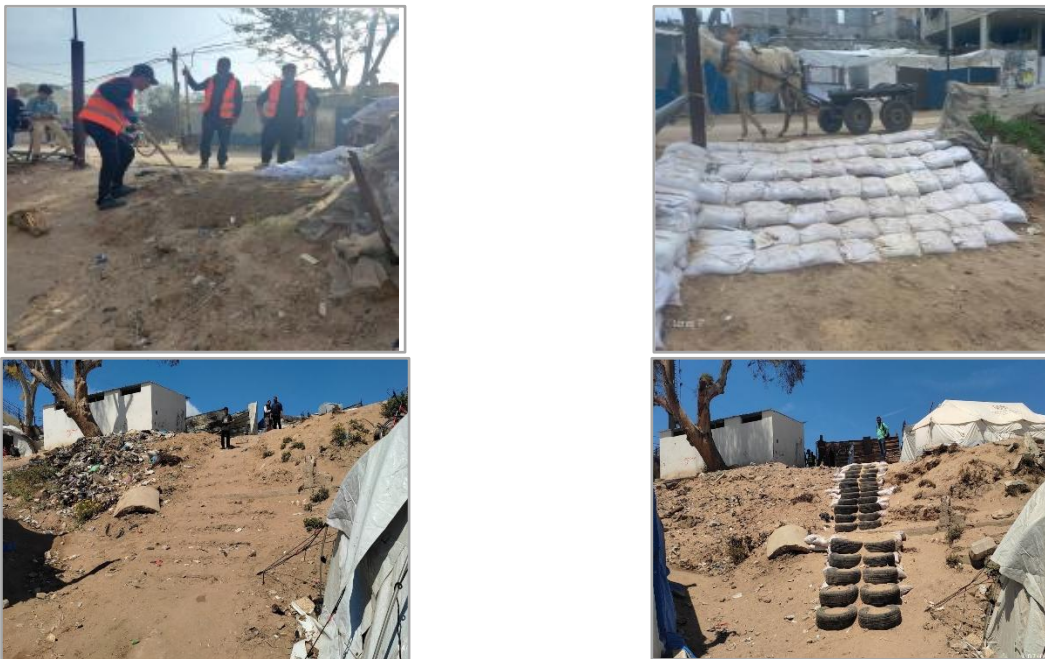
Figure1 Road leveling to facilitate access with local materials (Source: Humanity and Inclusion June 2025)
